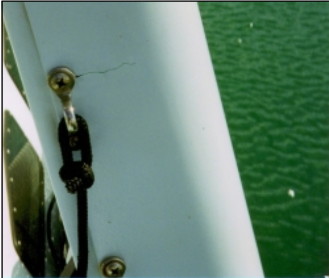
This beam shows a vertical crack that may eventually develop from a vertical flange glue line failure if not seen and repaired early enough - now it becomes more serious
